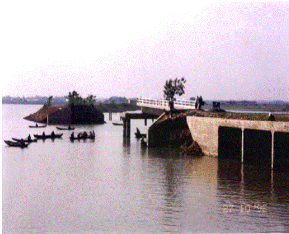
Photo 2 Damaged 67m bridge during 1998 flood on Turag-Bhakartha road near Amin Bazar
